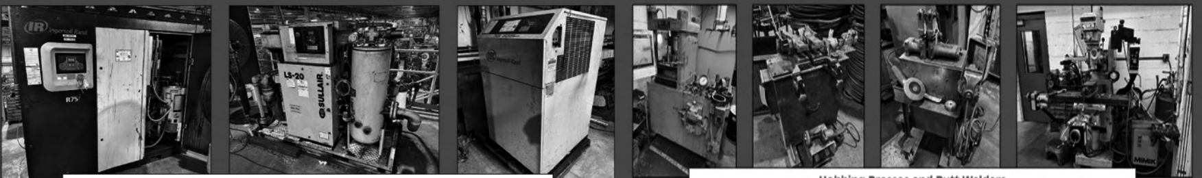
100-HP Ingersoll and Sullair Compressors
