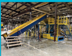
60" Diameter Densifier, 298 kW Motor
