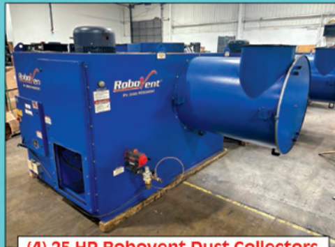
(4) 25 HP Robovent Dust Collectors (2016)
